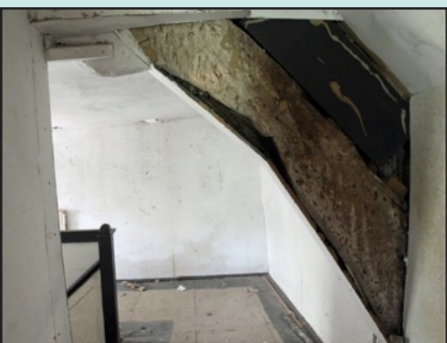
TOP RIGHT: The derelict Studley Grange farmhouse, Lydiard Tregoze. © Wiltshire Buildings Record.
